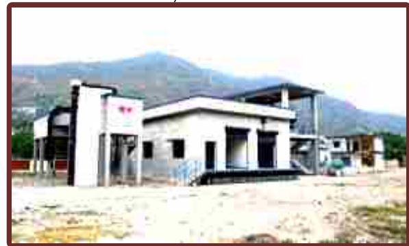
3.5 MLD STP AT SRINAGAR
